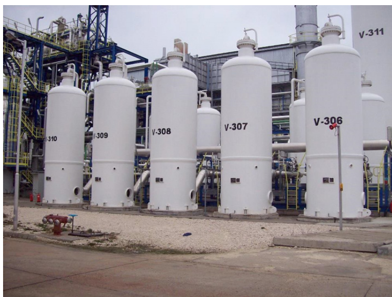
Figure 3. Hydrogen production plants: corrosion occurred because hydrogen bonded with carbon in the steel. Through fault detection analysis, MOL was able to get uptime back to 97%.
